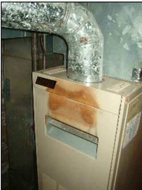
9. Evidence of furnace backdrafting
