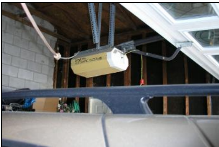
20. Extension cord for west garage door opener
