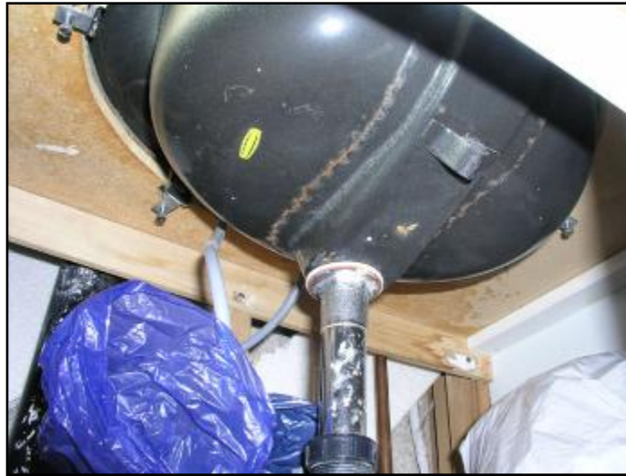
19. Steel basin rusting at weld
