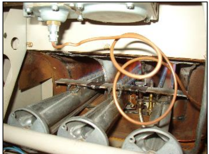
10. Rust at bottom of heat exchanger
