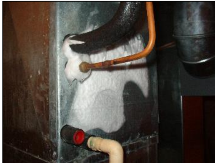
14. Frost visible on ductwork at AC coil
