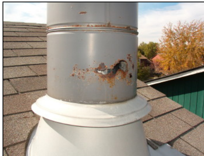
13. Rusted chimney wall from fireplace
